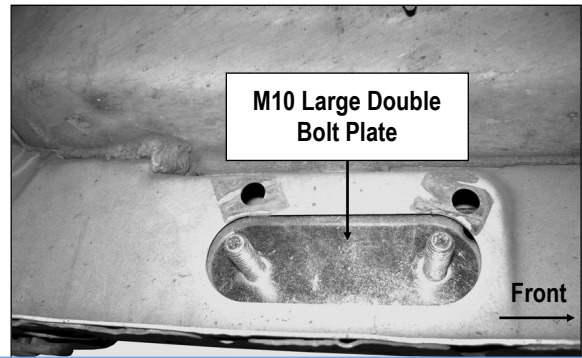
(Fig 3) M10 Large Double Bolt Plate Installed (On Driver Side Front Mounting Location)
