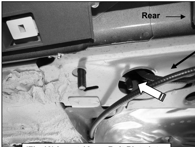
(Fig 19) Insert 10mm Bolt Plate into large hole and out smaller hole
