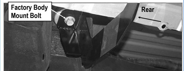
(Fig 8) Passenger Rear Mounting Bracket (PRM) Installed
